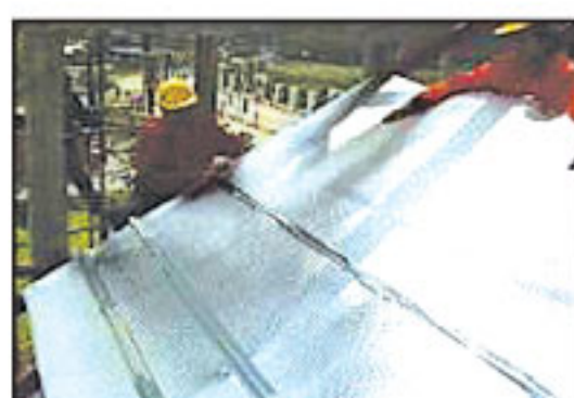
Step 5 Batten can be installed on top of CoolMax™ following the roof profile spacing.
