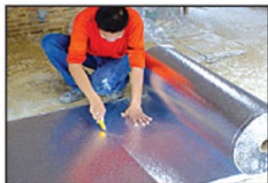
Step 1 Measure the width of the roof and by using blade cut the length accordingly.
